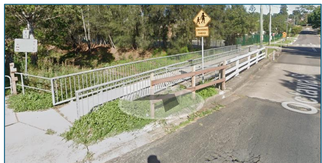
Google streetview image of the parallel bridge alongside Octavia St across Girraween Ck between Cumberland & Blacktown LGAs.
