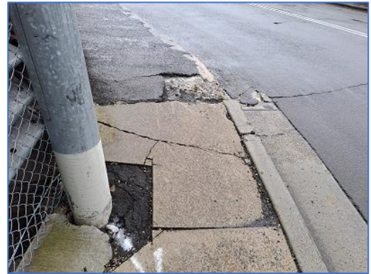
Damaged footpath from bridge turning left into Church St.
