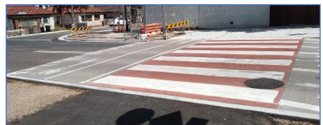
Combined Pedestrian and Cycle Crossing when under construction on Adderley St West, Auburn
