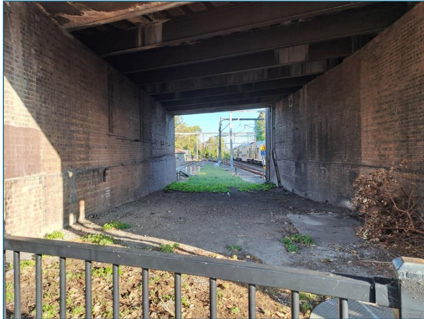
Current view from the end of Platforms 1 & 2 through to the south side of the existing bridge.
