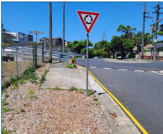
One 'pad' of wider concrete. Is this considered a 'shared path'?
