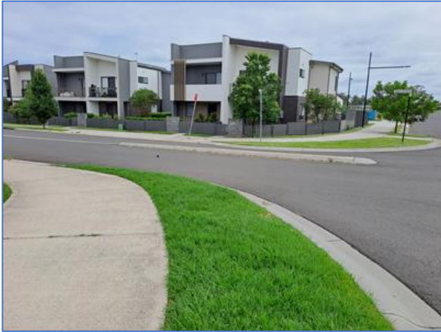
It may be hard to see with this photo, but at the corner of Calder St and Rosetta Street Schofields there are 'roll gutters' with no proper crossing. The other intersections along the Calder Street shared path have proper crossings.
