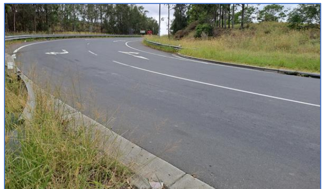
Crossing M7 northbound exit ramp (Points F to E on above image).
